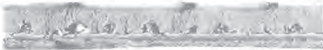
FIGURE 9 — This butt joint had a manual weld on the back side. Penetration came to within \frac{5}{32} " (4.0 mm) of the back-up bead and porosity resulted.
